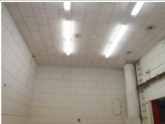
Photo #480 Makeup Air / Ventilators – None
