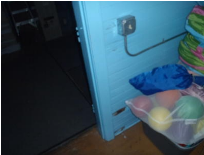
Photo #524 Wood Deterioration –
