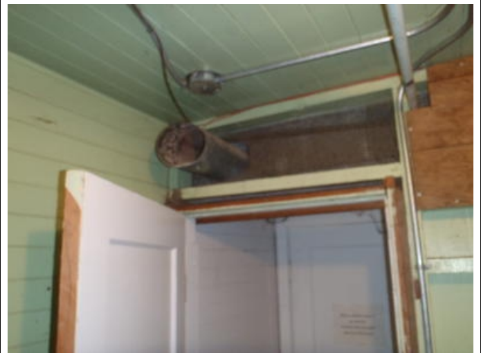
Photo #516 Makeup Air / Ventilators – None
