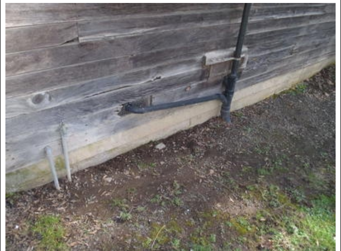
Photo #240 Water & Waste Pipe – Copper & ABS
