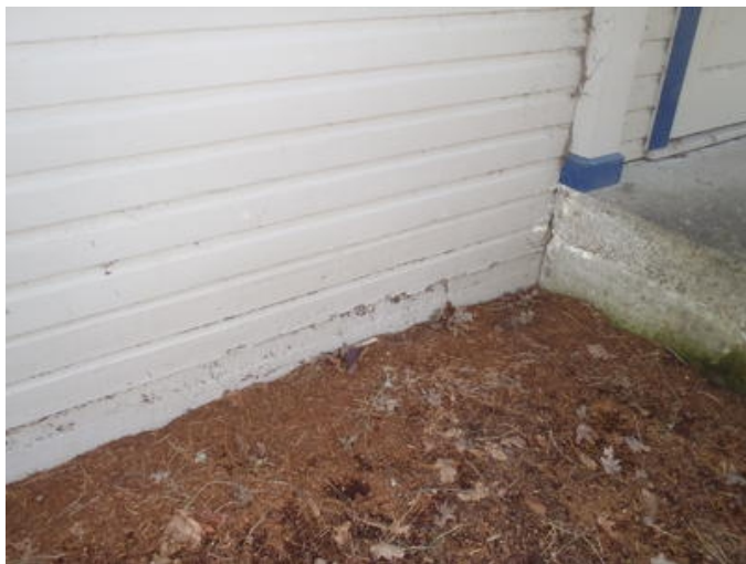
Photo #354 Siding Condition – Lapped Wood
