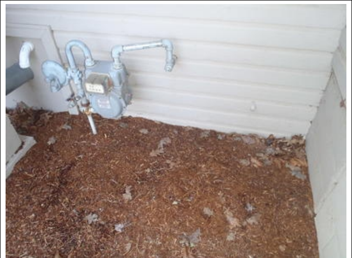
Photo #395 Siding Condition – Lapped Wood
