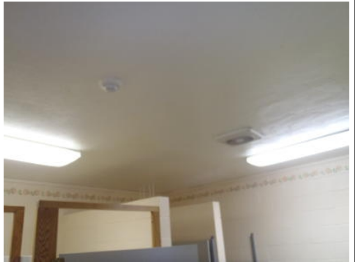
Photo #458 Ceiling & Wall Condition - Classroom &
