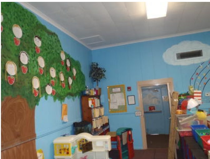
Photo #575 Ceiling & Wall Condition - Classroom &
