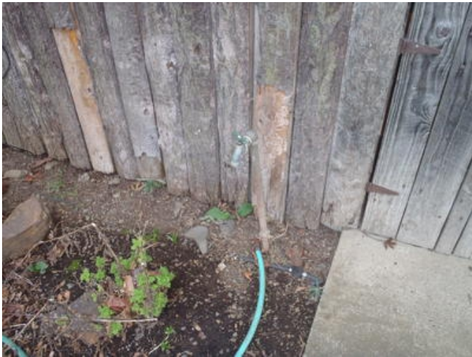
Photo #306 Siding Condition – Lapped Wood
