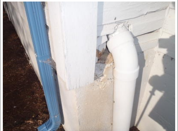
Photo #367 Siding Condition – Lapped Wood
