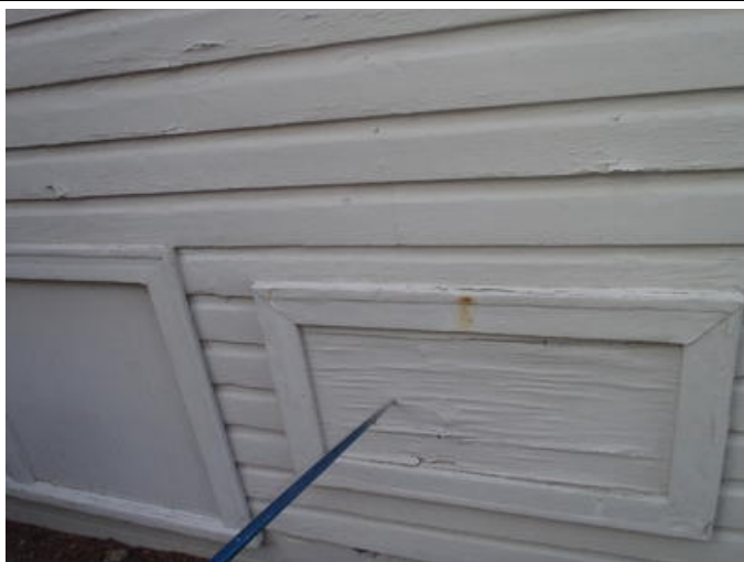
Photo #390 Siding Condition – Lapped Wood
