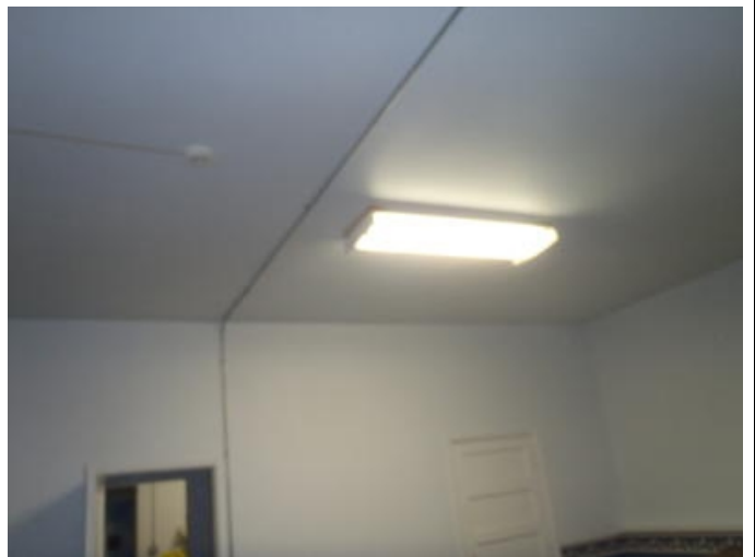
Photo #530 Ceiling & Wall Condition - Classroom &
